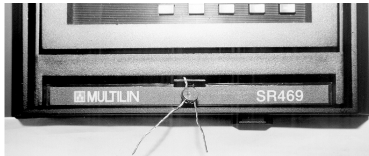
Figure 2-2: SEAL ON DRAWOUT UNIT
